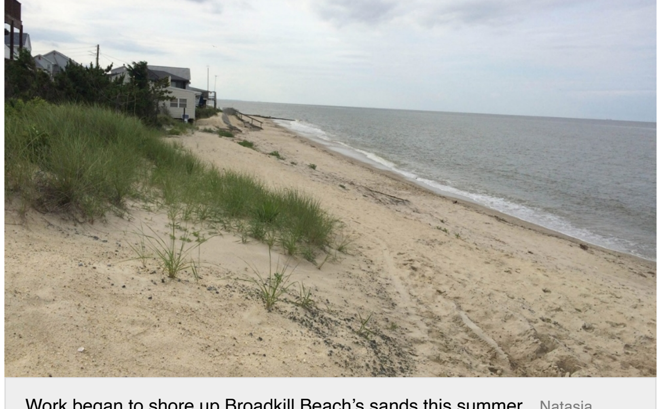
Work began to shore up Broadkill Beach's sands this summer. Natasja Sheriff
